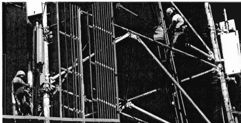
Technicians install antennae on existing towers throughout the GRADD region, which will bring high-speed wireless Internet service to residents of the predominantly rural region.
